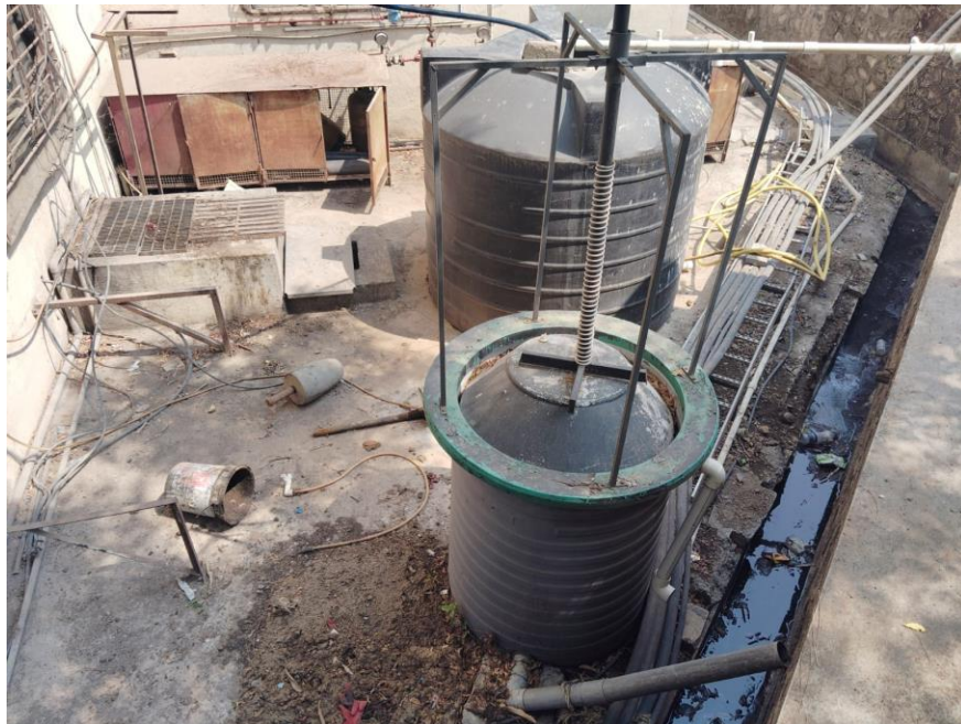
Bio-gas plant: Manages the organic waste and generate energy
